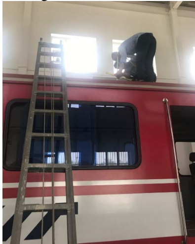
Fig. 1 GPS antenna installation
